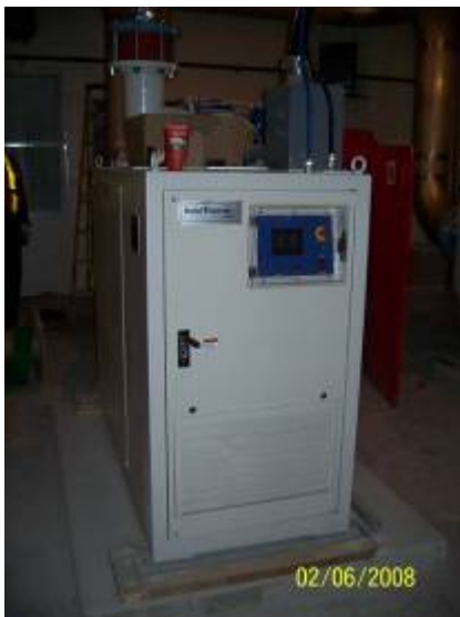
BAF Facility: The Neuros Blower shown above is a new high efficiency unit that will provide aeration of the BAF cells about 40% more efficiently than other available technologies..
