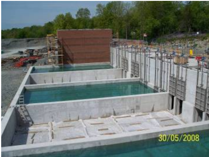
BAF Facility: This secondary treatment facility will remove more nutrients and dissolved contaminants from the sewage resulting in cleaner effluent to the lake. In the photo, some of the cells are being leak tested to ensure they are water
